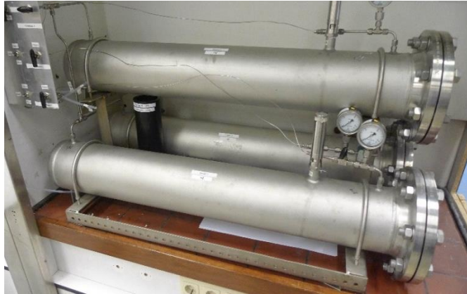
Figure 2: Cylinders filled with hydrogen at 2 bar
