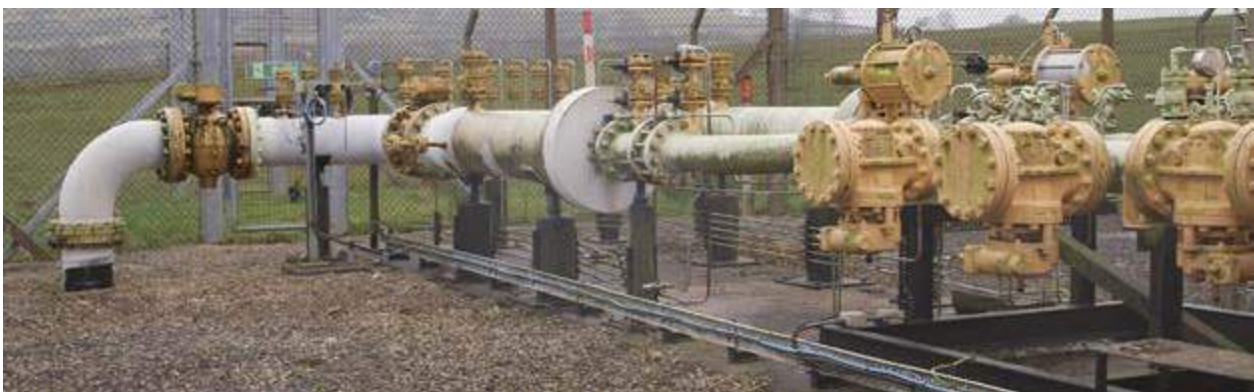
Image 10.6. 'Typical' Pressure Reduction Station (PRS)
