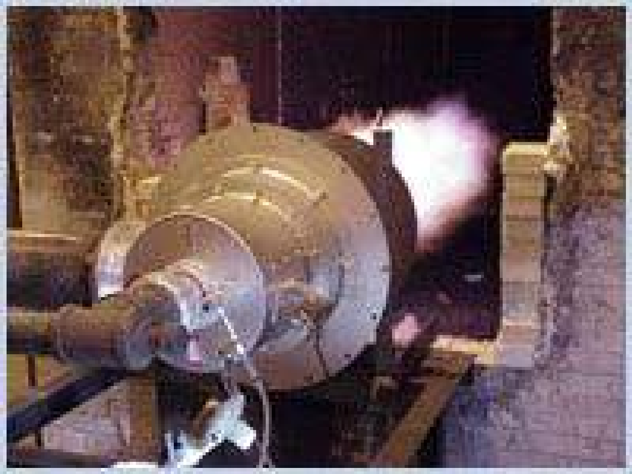
Image 5.9. MAXON Wide-Range (R) Burner Running on Hydrogen. (Source: https://www.maxoncorp.com/Directory/product/WIDE-RANGE-Burner/38/Natural-Gas-Burner-High )
