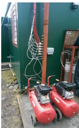
Figure 10: Compressors and vent stack
