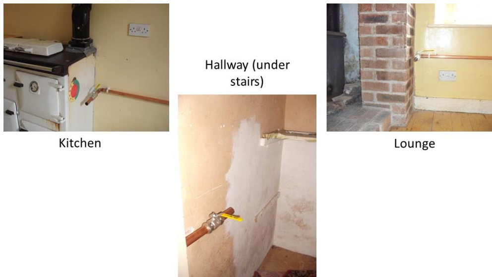
Figure 8: Gas injection points
