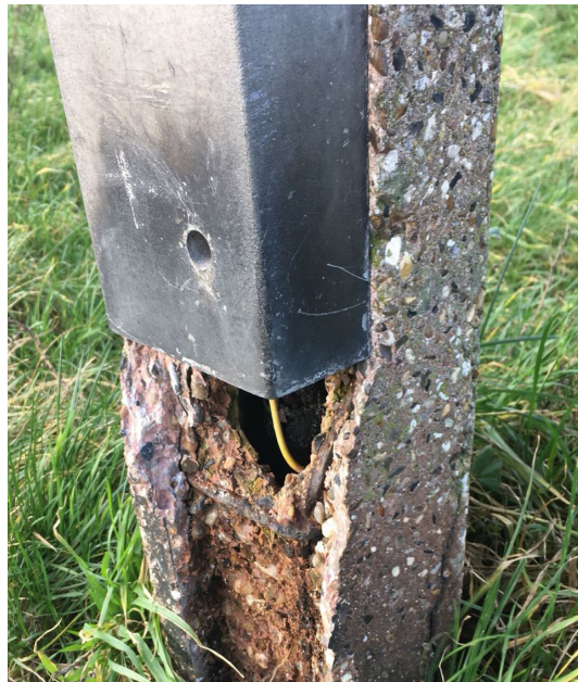
Exposed reinforcement due to frost damage.
