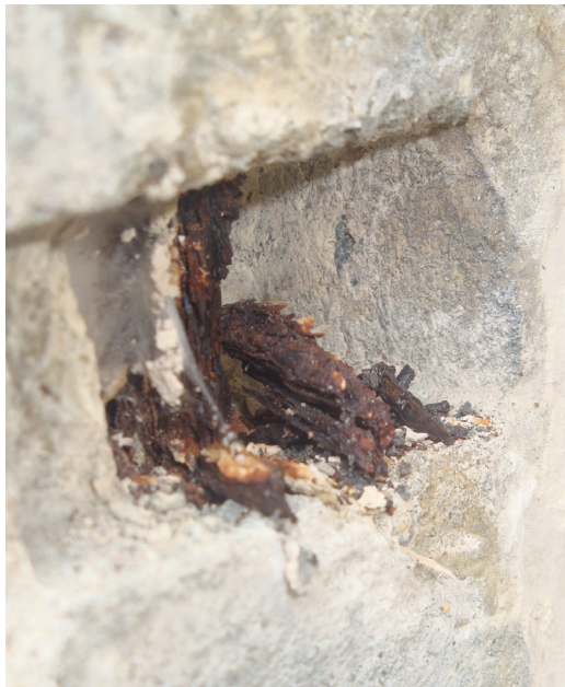
Missing mortar plug resulting in corrosion of reinforcement.
